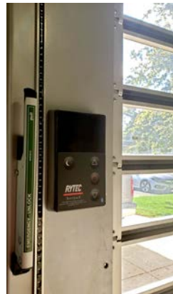
BTA4 Controller side column mounted
