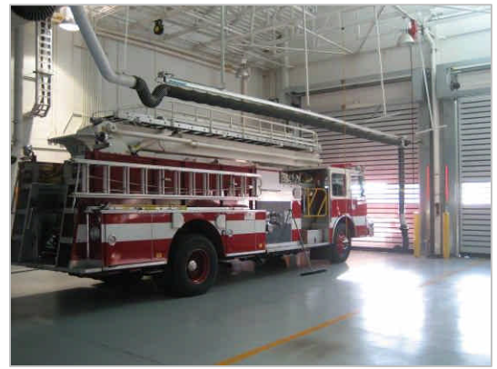
▲ Secured in Station. Fire truck secured behind the rigid door panel consisting of interconnected slats with reinforced hinges.
